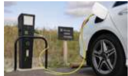
Electrical Charging Point
